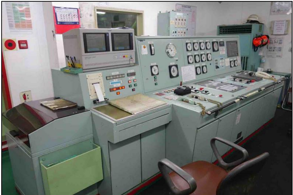
Figure 3: Engine Control Room
