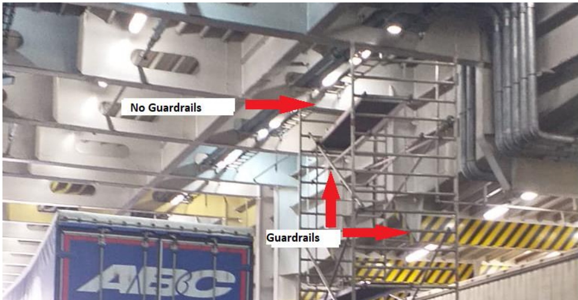
Picture 14: Top of Mobile Scaffold where Workers Work
