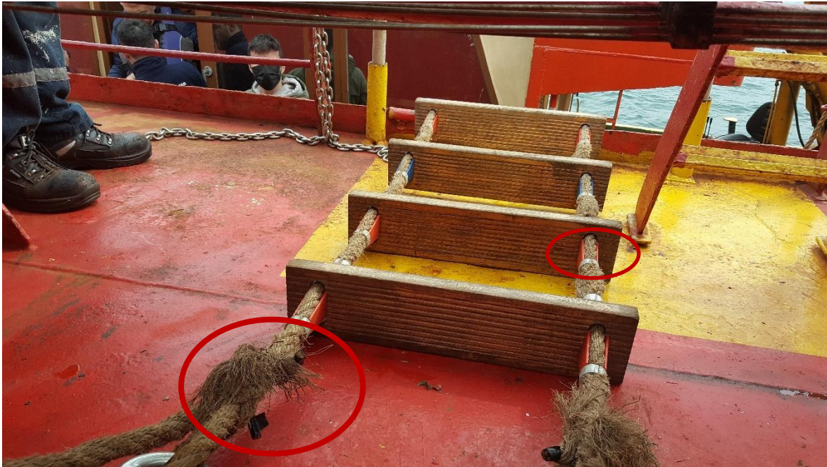
Image 16 General condition of the step of the side ladder
